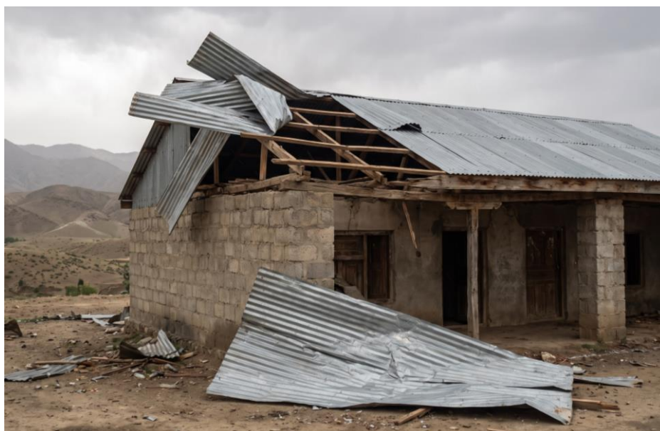
Figure 8.2 Wind loss of profiled roof sheets initiating at the roof edge
