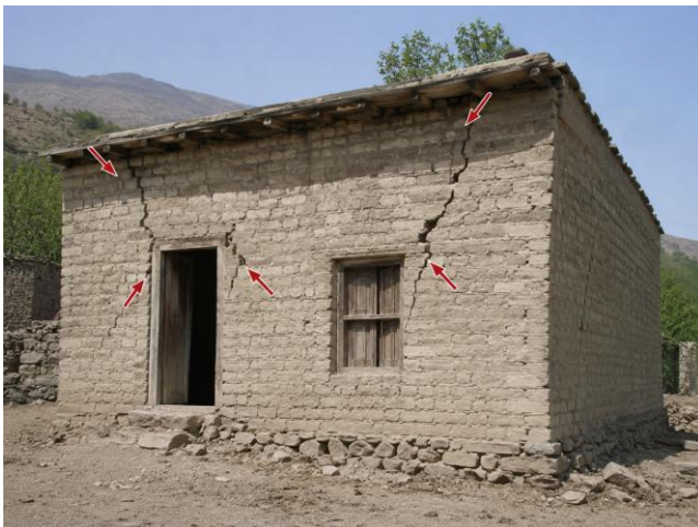
Masonry without confinement with diagonal cracks originating from the openings
