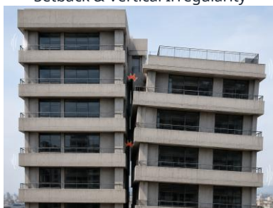
Inadequate Separation/ Ponding
